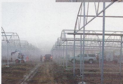
Fog, rain and high winds made construction on BFN's new structures challenging.
