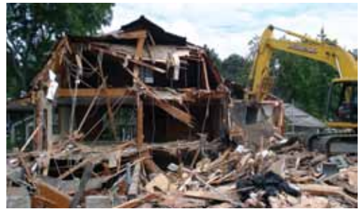
Briggs Nursery decided to do a full rebuild, which meant the old building had to go.
